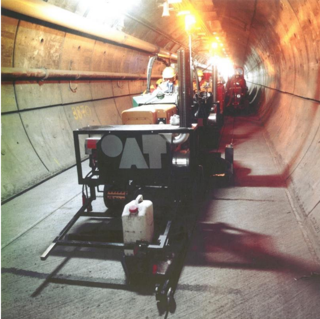
The Channel Tunnel has been connecting France and Great Britain for 30 years. The performance grout PCI Vergussmörtel 50* was used to fill the cable grooves in the service tunnel. ( Link to high-resolution photo)
